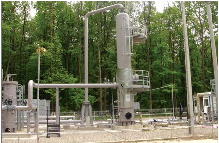
Accurate and reliable delivery of recovered glycol (TEG) to the top of the absorber vessel is critical at this final stage of gas drying.
