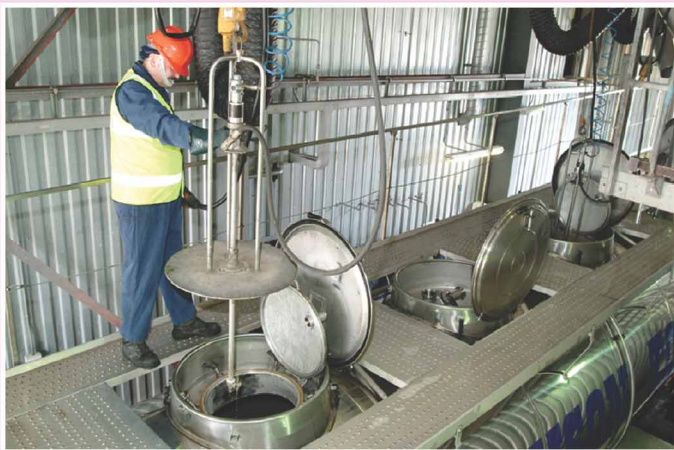
One of three Spraying Systems automatic tankwash units is lowered into working position at Atchison Topeka. The Hydra-Cell G35 seal-less pumps feeding these units with hot liquid at 70 bar pressure are still in daily use after six years service
